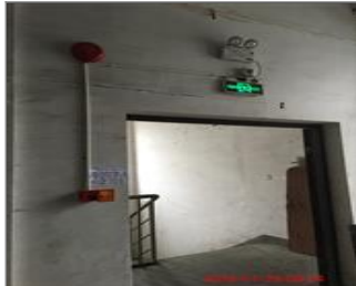
Photo of fire safety equipment Exit sign and emergency light and fire alarm.JPG
