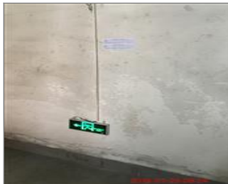
Photo of fire safety equipment Evacuation sign.JPG
