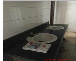
Photo of the sanitary facilities Basic supply provided in toilet.JPG
